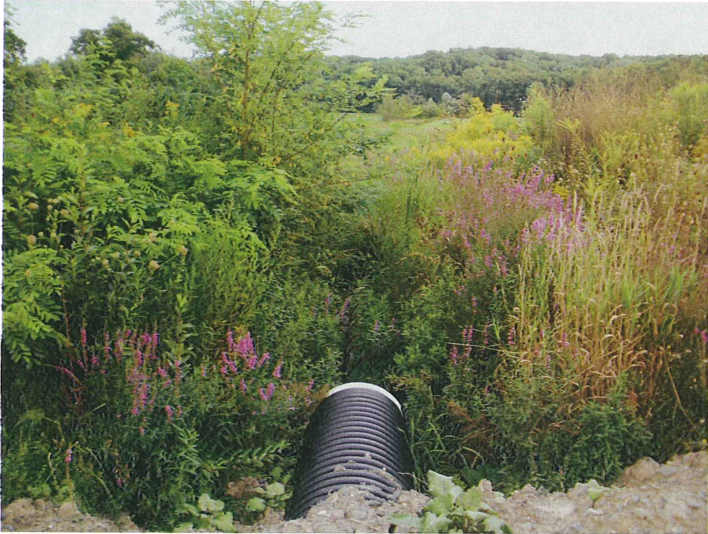
Photograph of 24" pipe near northwest corner of property. August 24, 2011.
